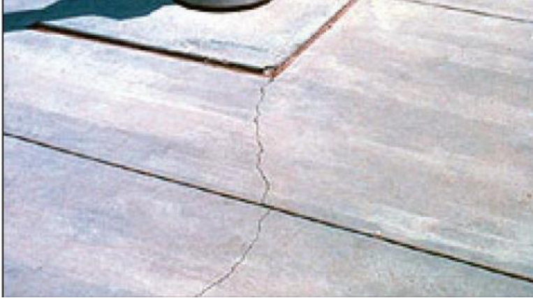
Plate 4- 3: Drying shrinkage cracks (Texas Department 2006).
