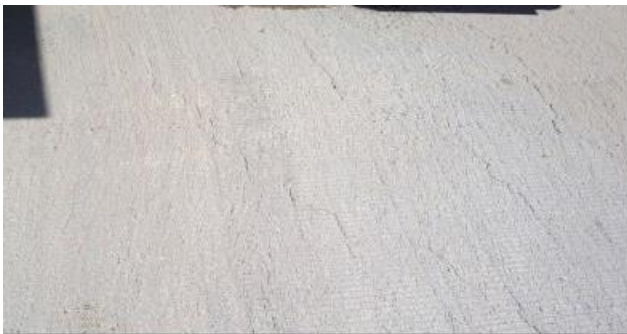
Plate 4- 1: Shrinkage cracks (Handojo 2009).
