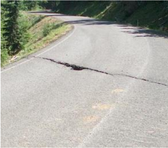
Figure 1.2 sub-grade failure cracks
