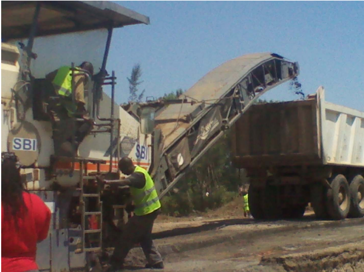
Figure 2:A milling machine grinding and collecting the milled RAP at Kericho-Nyamasaria road (SBI)
